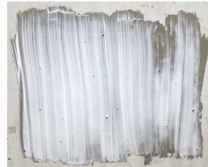
Iso-Tek™ 8501 Gel applied to a 14,000 PSI vertical wall on 432 Park Ave, NYC.
